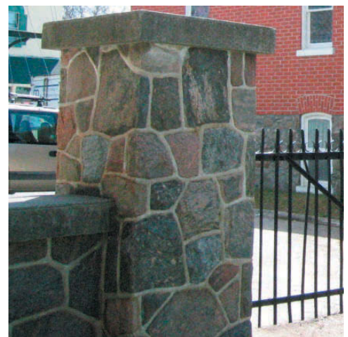
Figure 4.28 The existing stone wall on Main Street at the entrance to the Fairgrounds. A more durable natural stone retaining wall product should be used to maintain the look and feel of the original wall for when it needs to be replaced.
