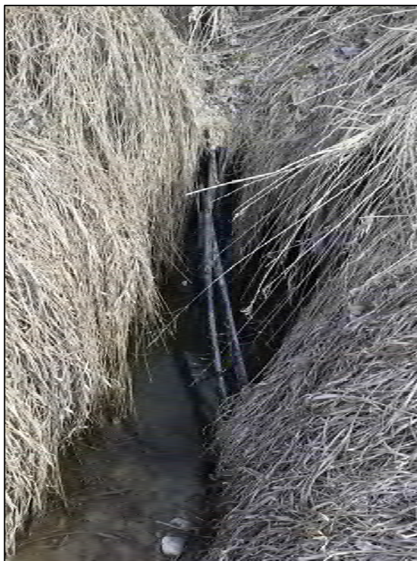
Photo 5: Exposed cables at HDF E, facing northeast (April 3, 2020)
